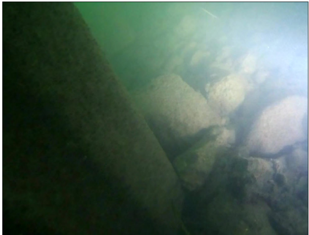
Pier 11w, footing exposure and channel bottom, typical
