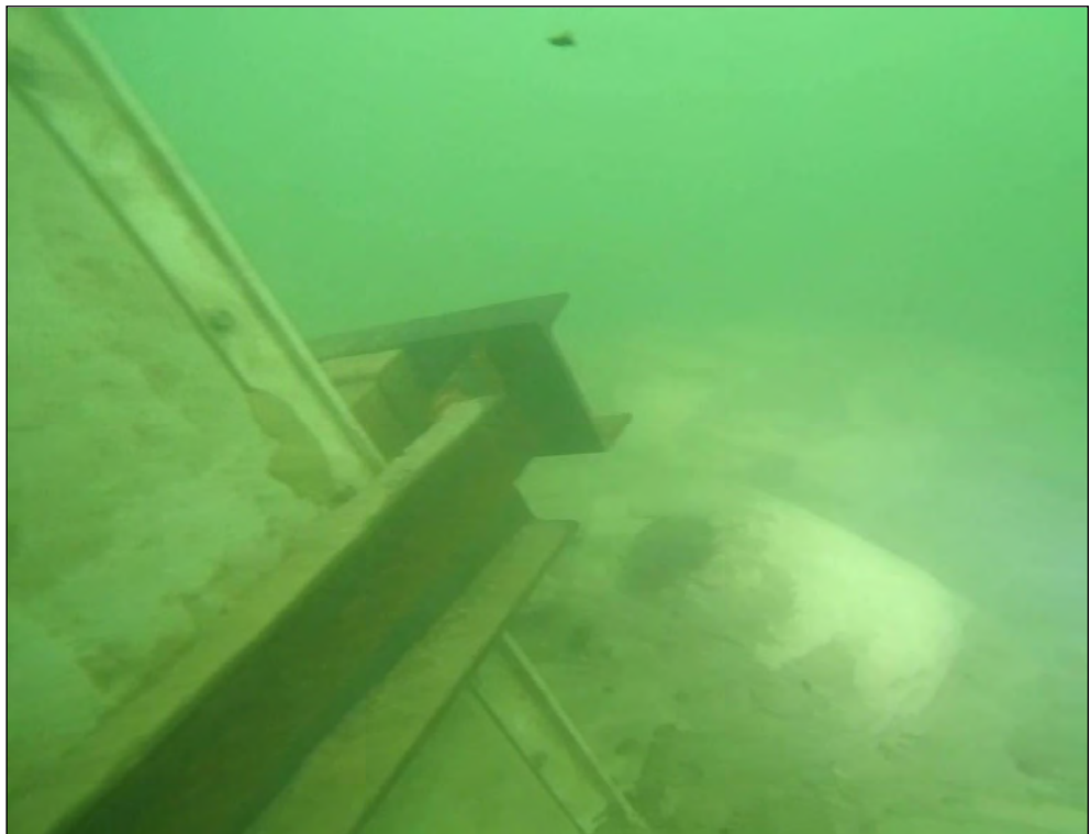
Pier 6w, corner of vinyl sheeting, steel walers and grout bags at channel bottom, typical
