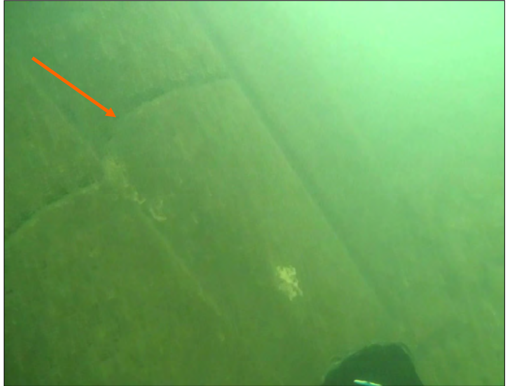
Pier 3w, horizontal crack in footing, typical west and east elevations
